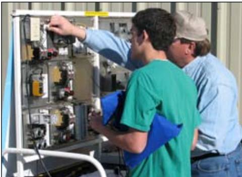
Tyson Maintenance Department allows students to experiment with a couple of their trainers they use in the plant to train maintenance employees.
