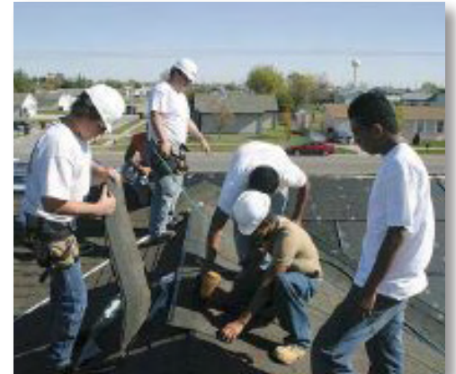
Students in the 2007-2008 ABLE Student Construction Class work on the roof of the home that is now complete and for sale on South Adams Street in the new CED addition. Listing agent: Patti Johnson BHA
